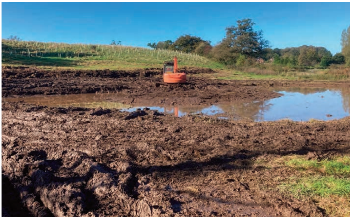
Figure 15: An excavator creating a large pond at the base of a slope, on which a woodland has been created. (©Sam Hope, Wyre Rivers Trust)
