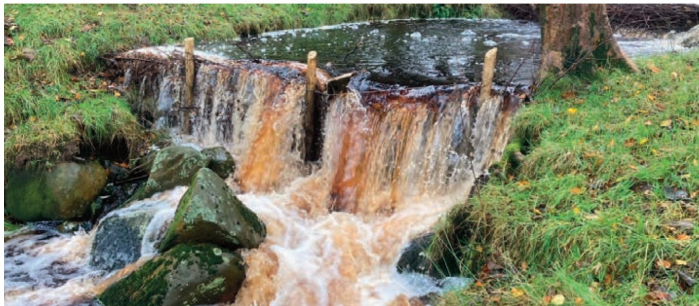
Figure 3: A leaky barrier in high flow conditions. A number of fascines (bundles) have been placed in the river to help slow the flow and store water behind the barrier during periods of heavy rainfall, helping to reduce downstream river levels. (©Sam Hope, Wyre Rivers Trust)
